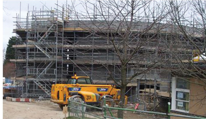
The 500-pupil Manor Community School currently under construction will include a 10m solar array
