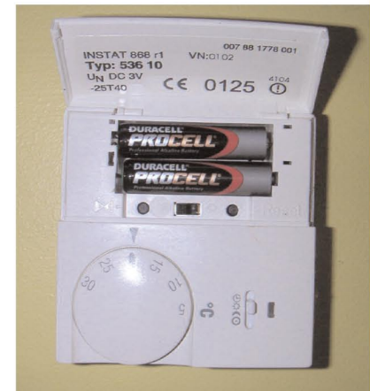
The batteries in this wireless thermostat have been fitted the wrong way round! So in effect there is no control...
